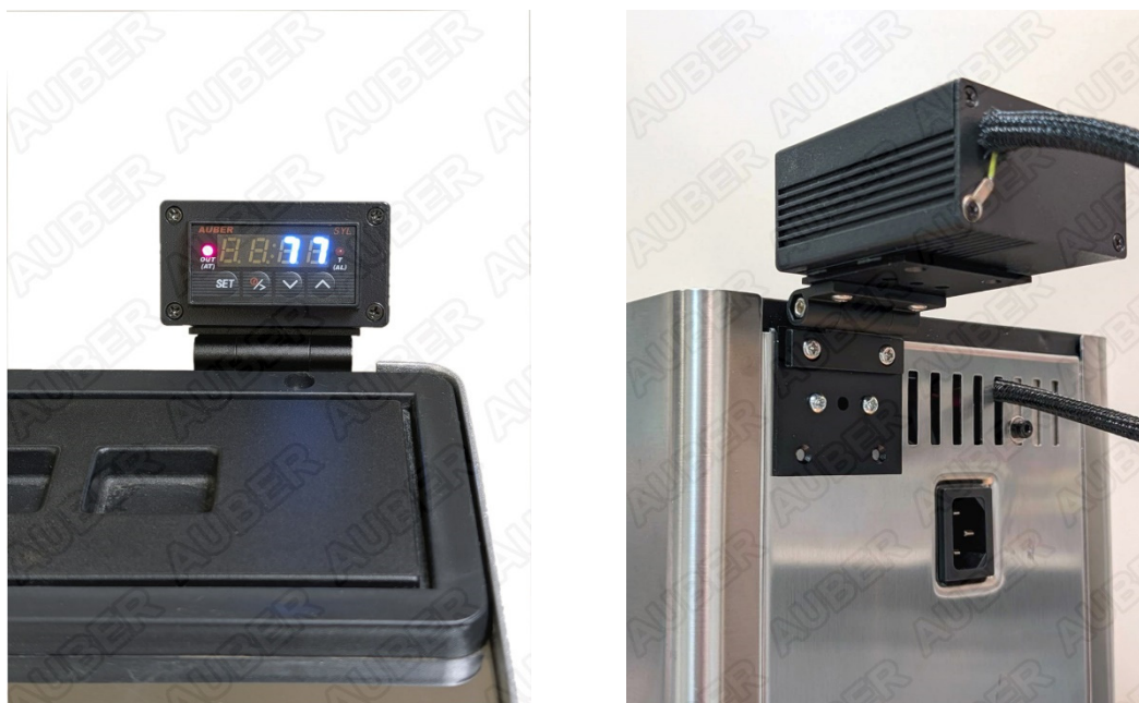
Figure 5. Front and rear view of the controller box mounted on the bracket.
