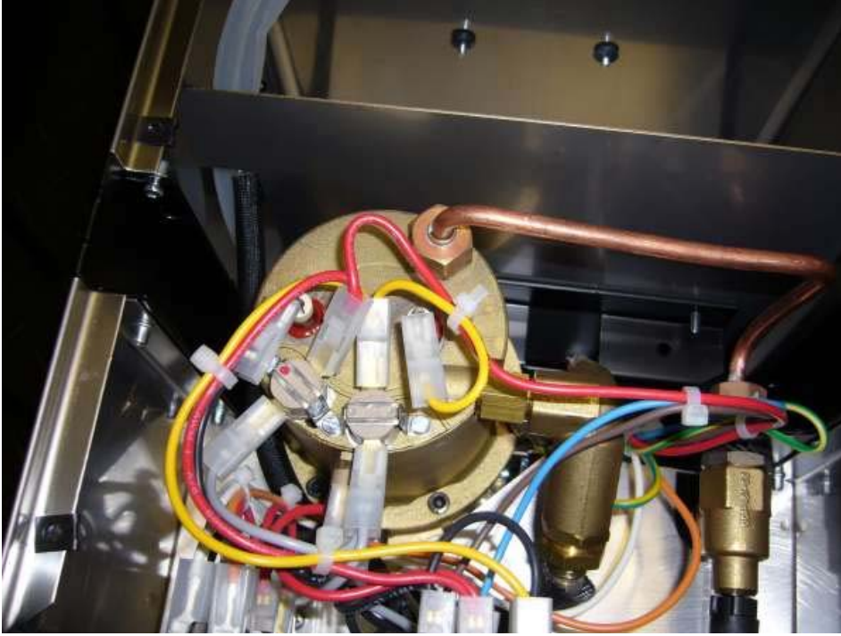
New boiler design after Aug 2006. Steam pipe now comes directly off the top of the boiler, overpressure valve is attached via a joiner fitting.
